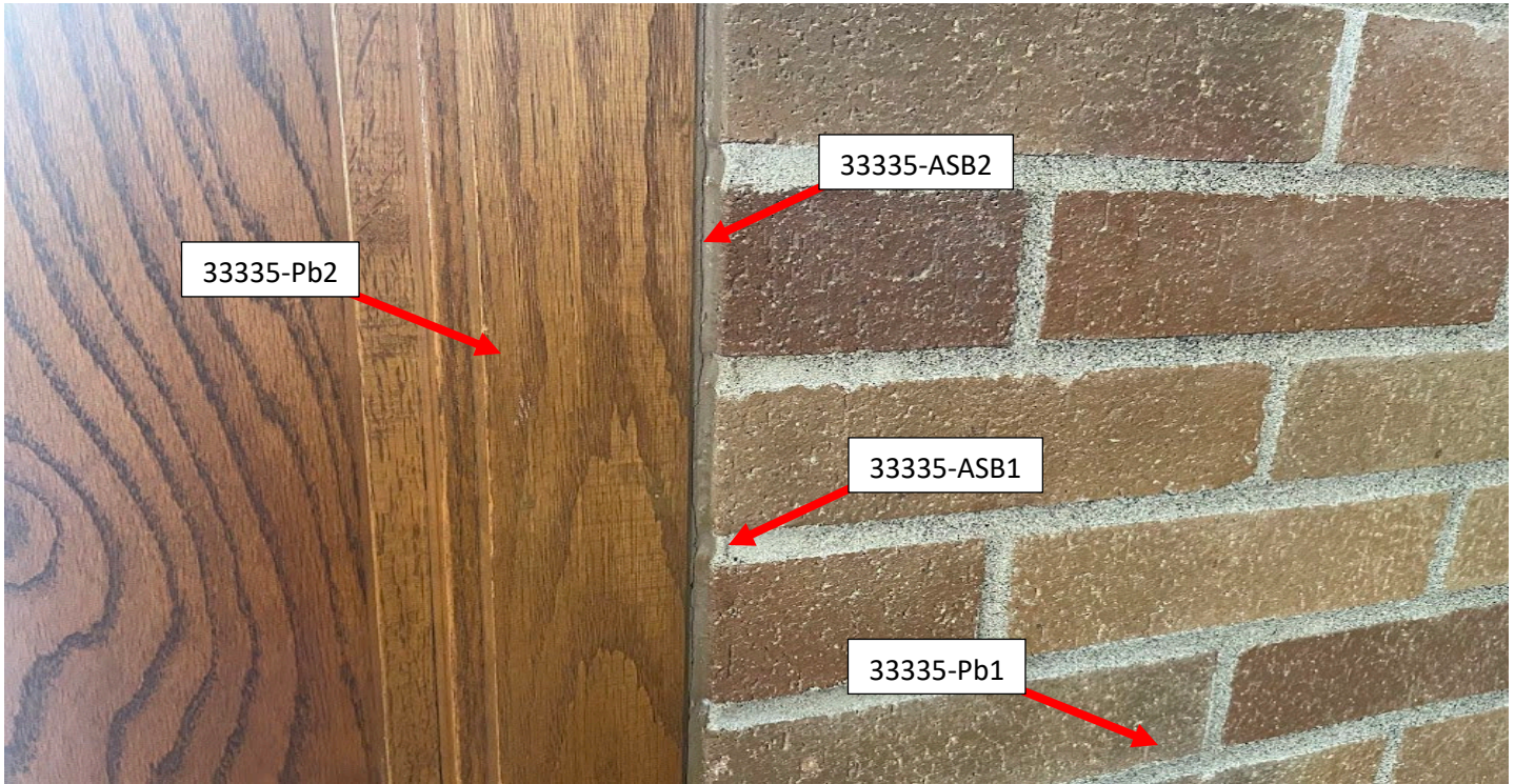
Pic. 1: Brick and mortar, Brown door caulking with gray foam backing & Brown door varnish
