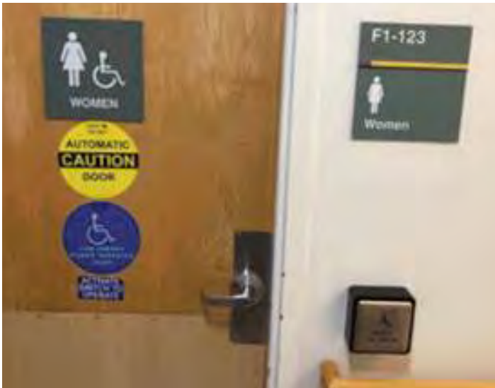
Figure 10.3.3-9. (PAD B100) This is an accessible restroom, but only the ID sign on the door shows that. The wall ID sign does not. There are too many signs regarding automatic door signage: three signs on the door, along with the push plate on the side. (It is unclear if these are all required by code.)
