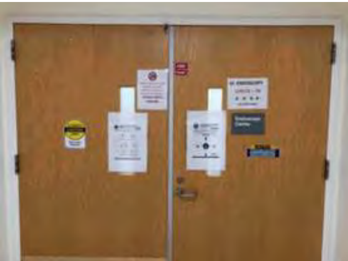
Figure 10.3.12-31. (PAD B100) This doorway to the Endoscopy Center is cluttered with so many signs that viewers are likely overwhelmed and unable to sort out the relevant information. The ID sign gets lost among the clutter.
