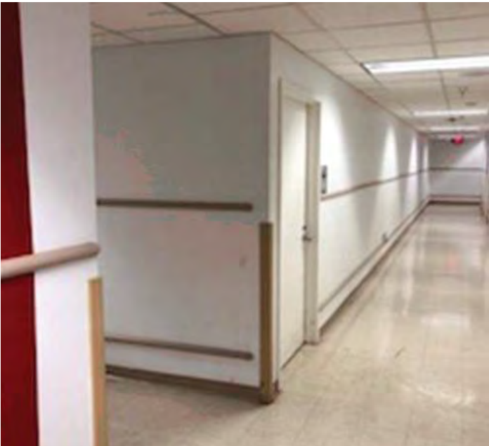
Figure 10.3.8-25. (MPD B334) The first corridor off the long hallway is not labeled by a ceiling-hung or projecting sign to indicate the functions found there.
