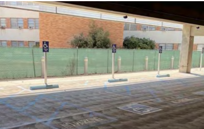
Figure 10.2.9-30. Markings at accessible spaces are difficult to see.
