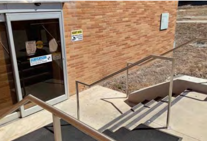
Figure 10.2.12-44. This entry door at the bottom of steps is missing a directional sign identifying an alternative accessible entrance.
