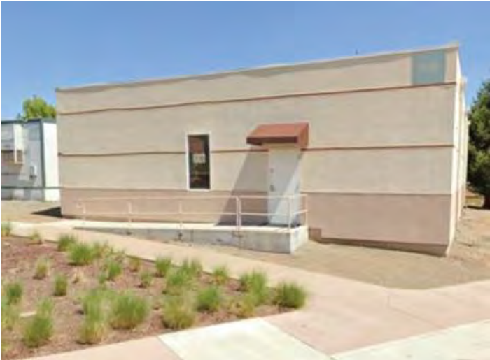
Figure 10.2.11-40. The faded, illegible building number at the top of Building 7D at PAD prompted staff to post an identification sign in the windows.
