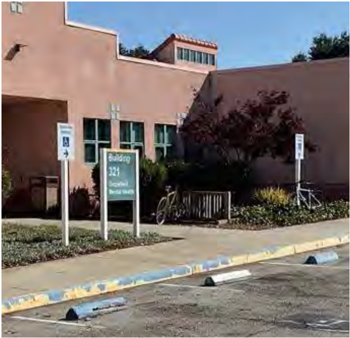
Figure 10.2.8-25. Without a curb cut, there is not an accessible route from parking to entrance.
