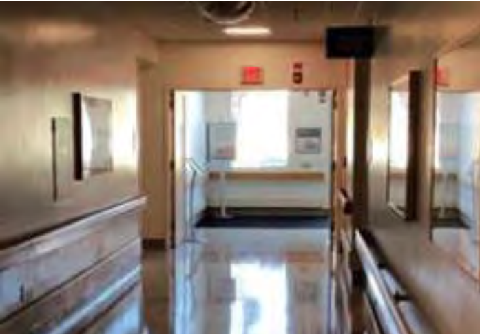
Figure 10.3.10-26. (PAD B100) This identification sign for Nuclear Medicine is ineligible due to back-lighting (a window) and the absence of dedicated lighting for the projecting sign.
